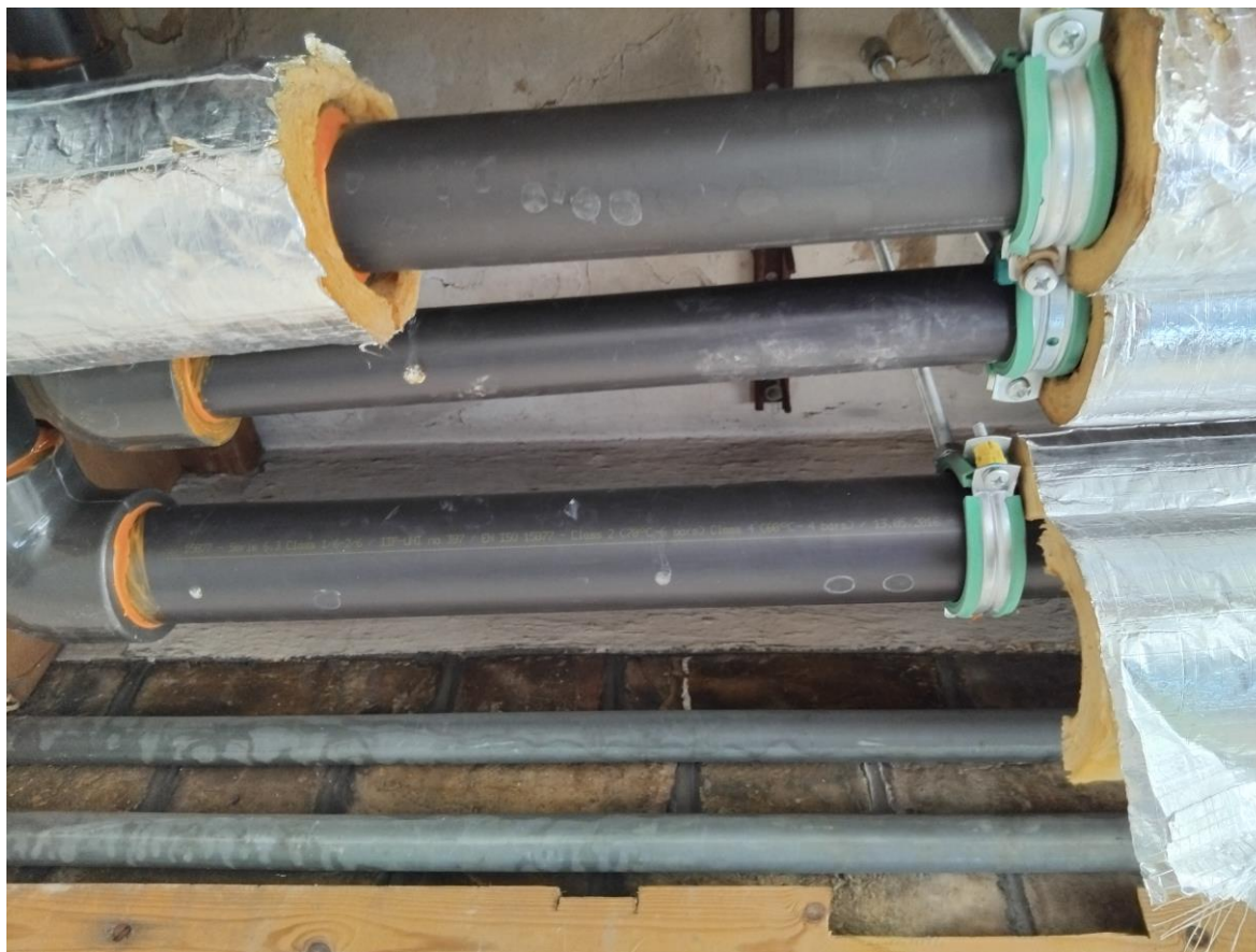
Figure 25: Plastic secondary network pipework leaving a substation
