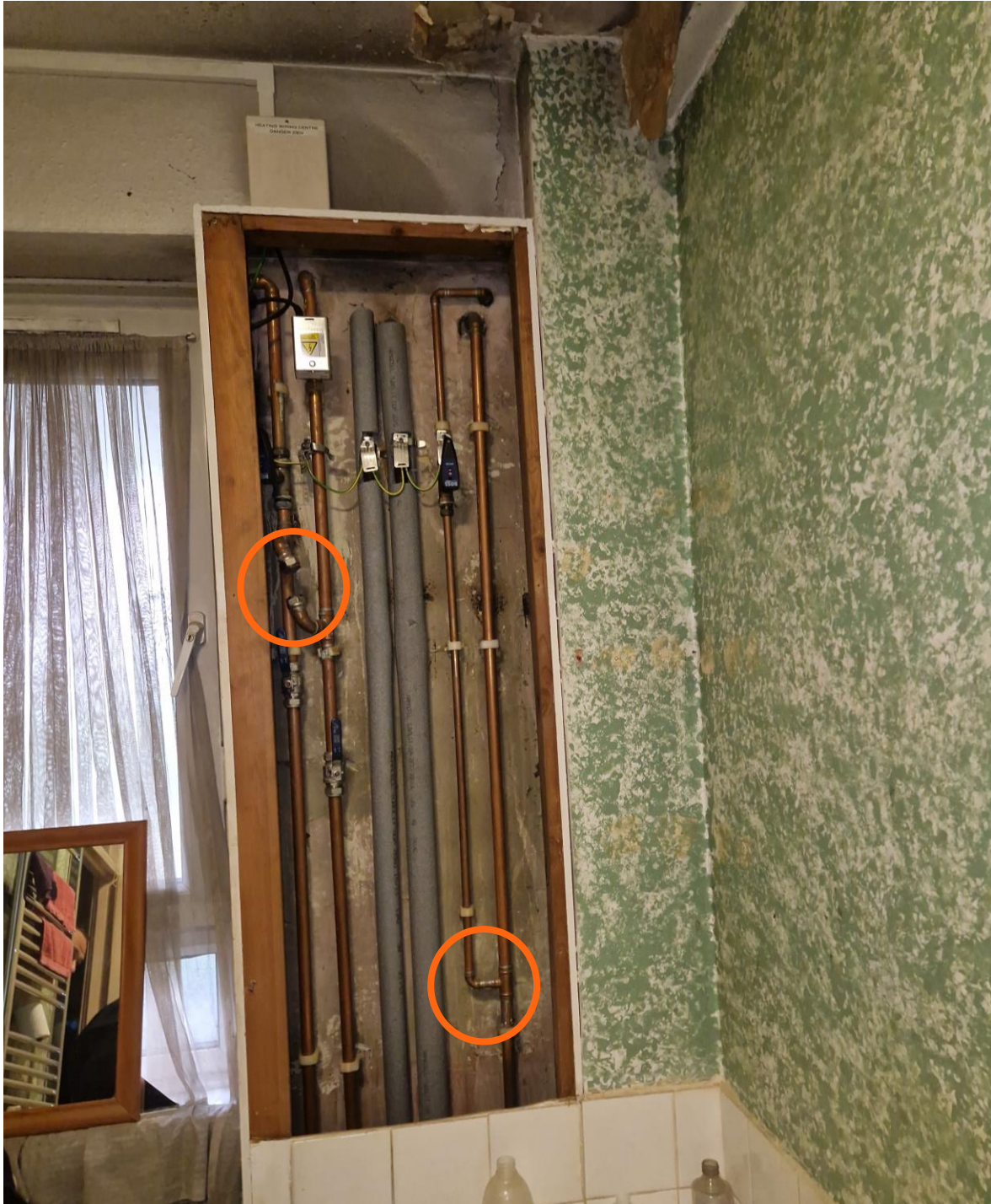
Figure 23: Fixed bypasses on DHW and space heating pipework behind wall panel, with one of the bypass legs removed (left)
