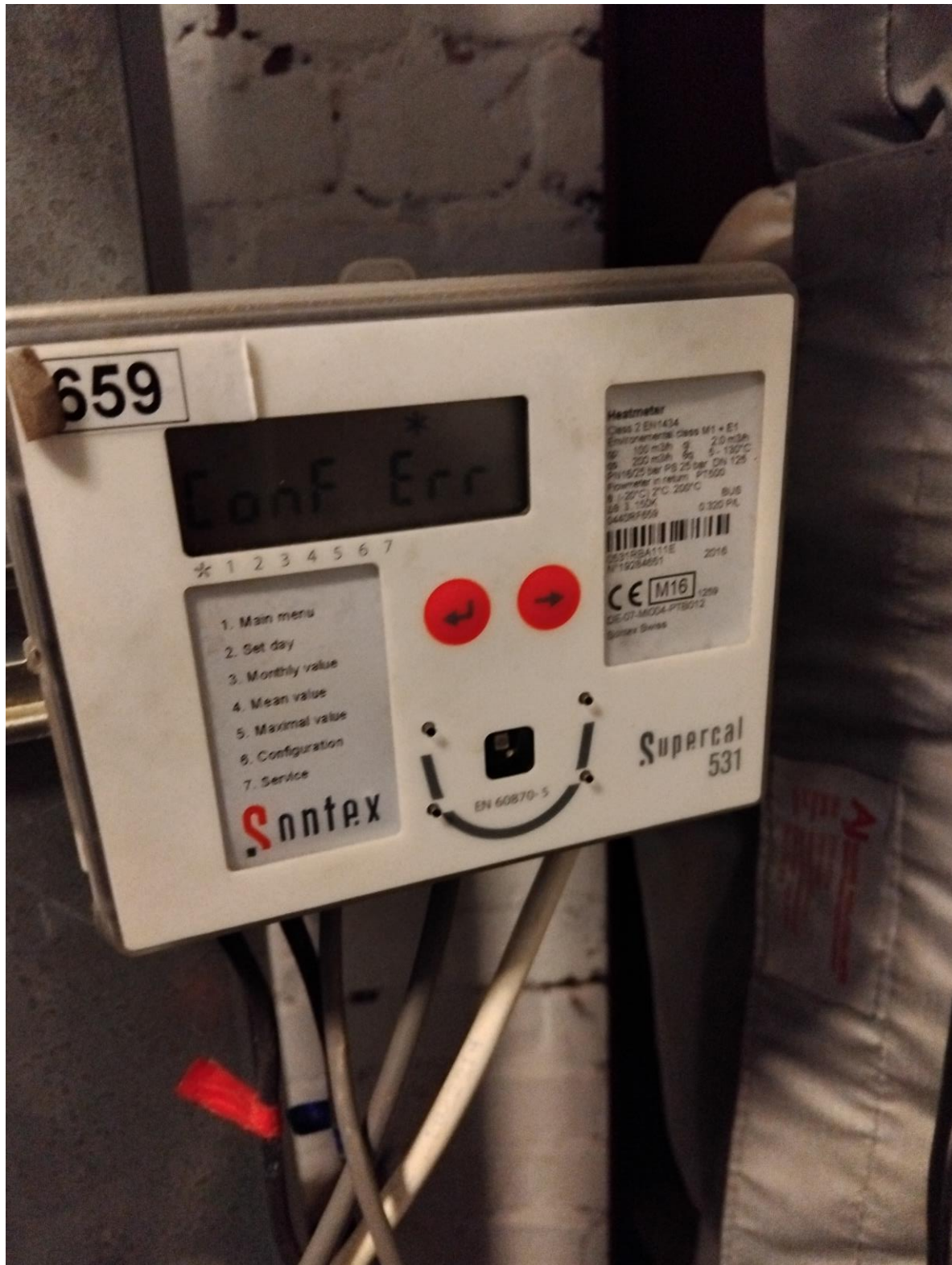
Figure 30: Heat metering installed but with errors preventing data reads
