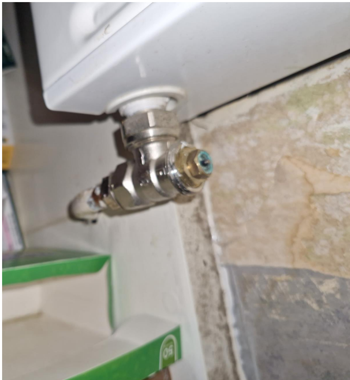
Figure 24: TRV with valve head/actuator removed, leading to reduced space heating control
