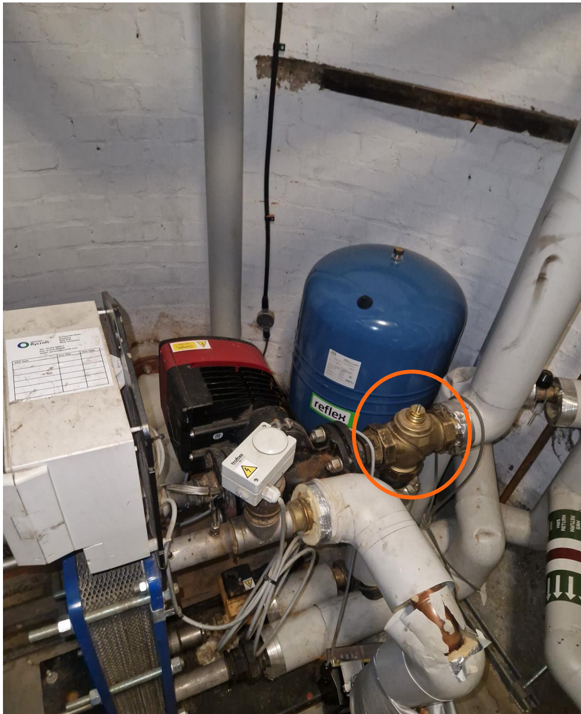
Figure 29: DHW plate heat exchanger with 3-port valve actuator missing
