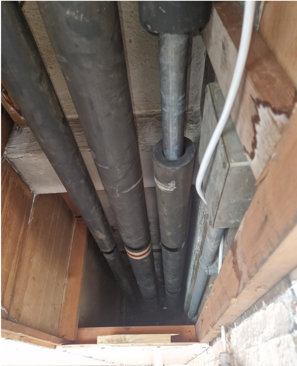
Figure 27: Nitrile rubber insulation on lateral pipework, with sections uninsulated
