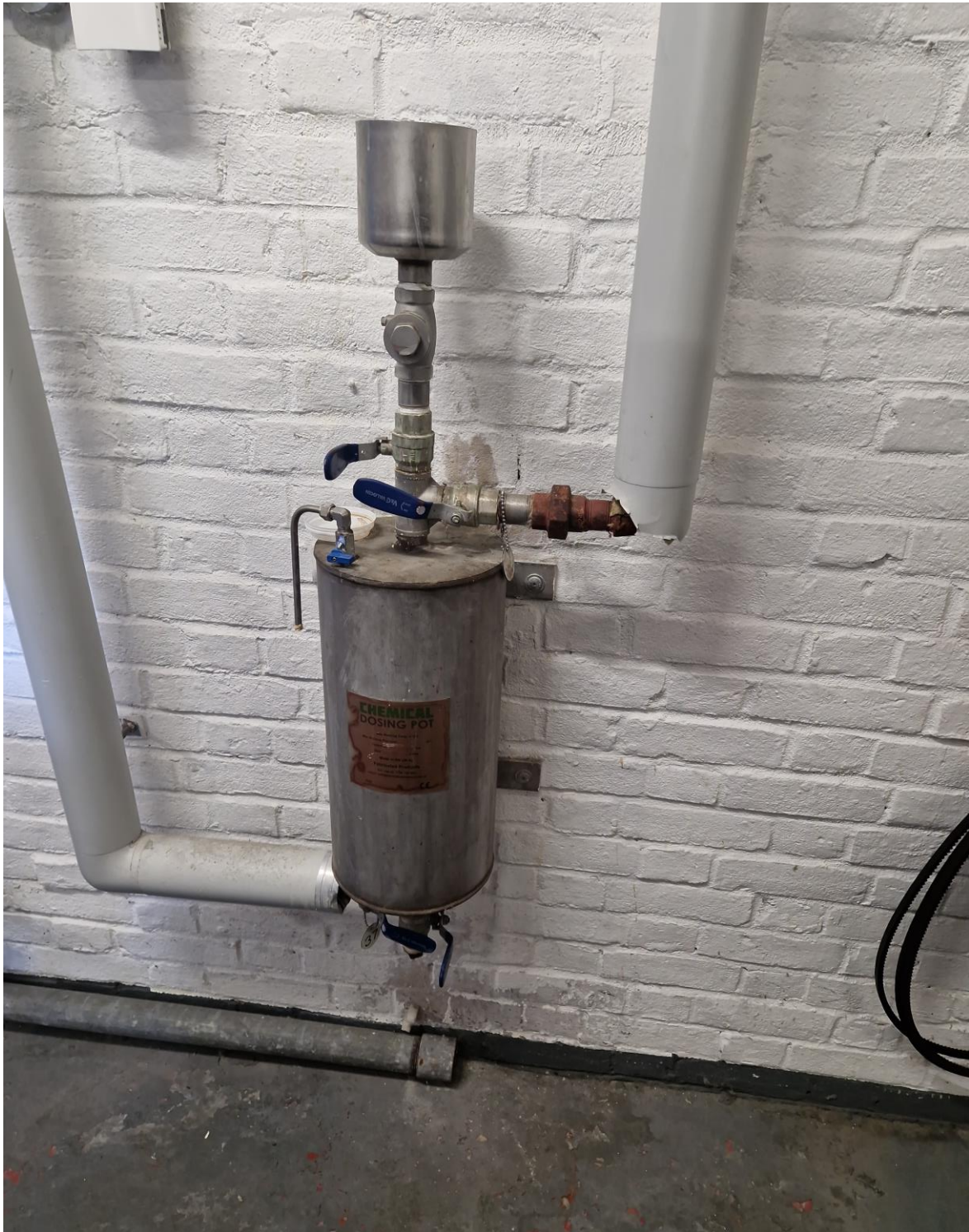
Figure 33: Dosing pot installed across flow and return pipework, creating a bypass leg (and a dead leg when isolated)
