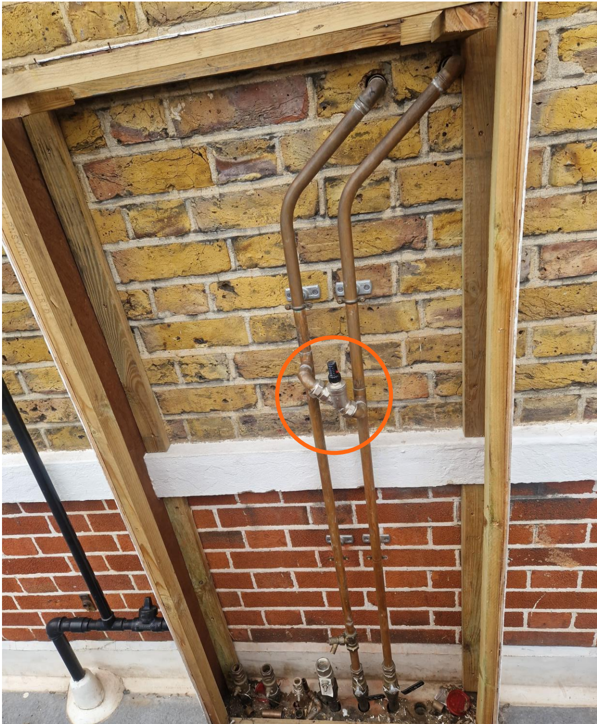
Figure 26: Fixed bypass on uninsulated external network pipework
