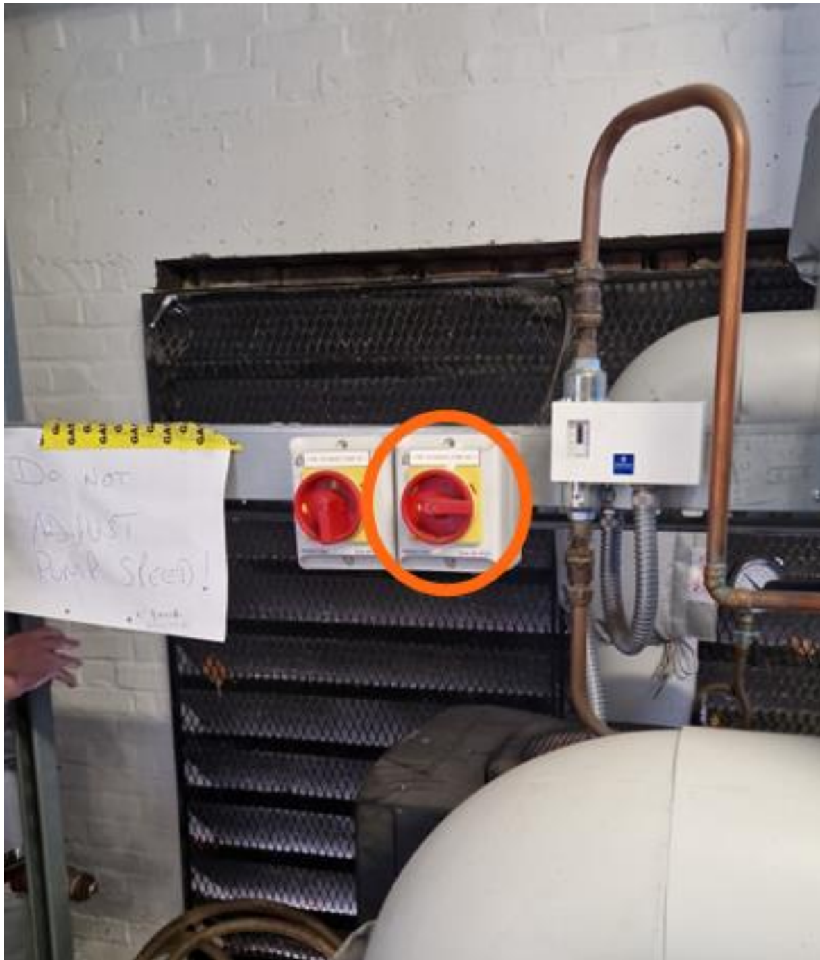
Figure 32: One network pump electrically isolated, leading to no redundancy
